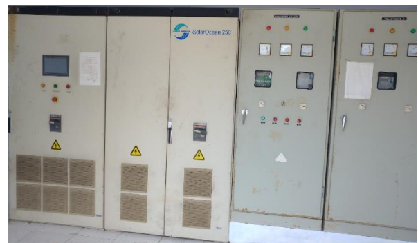
Fig. 3. Samil Power Solar Ocean 250 Inverter
