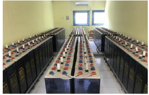
Fig 5. The Configuration of Battery Bank
