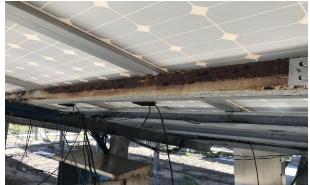
Fig 9. Photovoltaic Array Support
