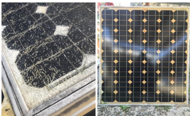
Fig 8. The condition of the photovoltaic module
