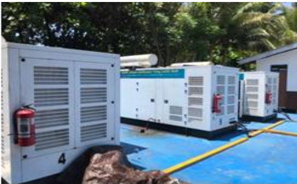
Fig 7. The Design of Diesel generators
