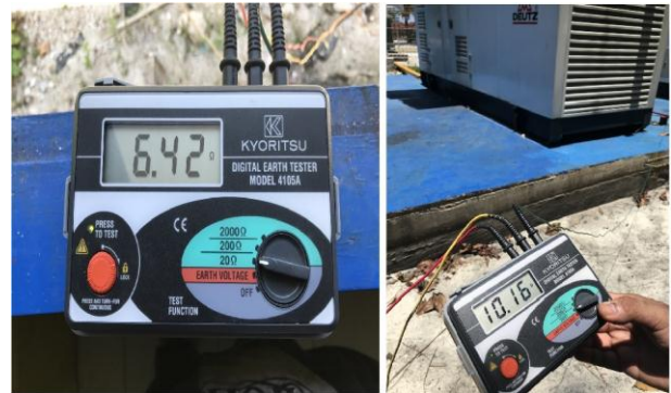
Fig 13. The measurement of the grounding system
